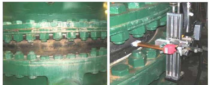
FIGURE 5: EXPANSION JOINT WITH SCANNING EQUIPMENT
